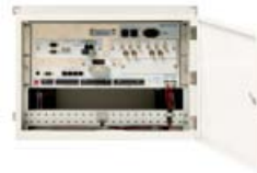
Data Acquisition Unit
